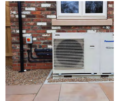
ref.14: Image showing Air Source Heat Pumps
